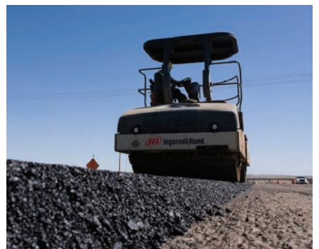
The New Mexico Dept. of Transportation's initial round of ARRA-funded projects is worth more than $106 million. (Photo courtesy NMDOT)
