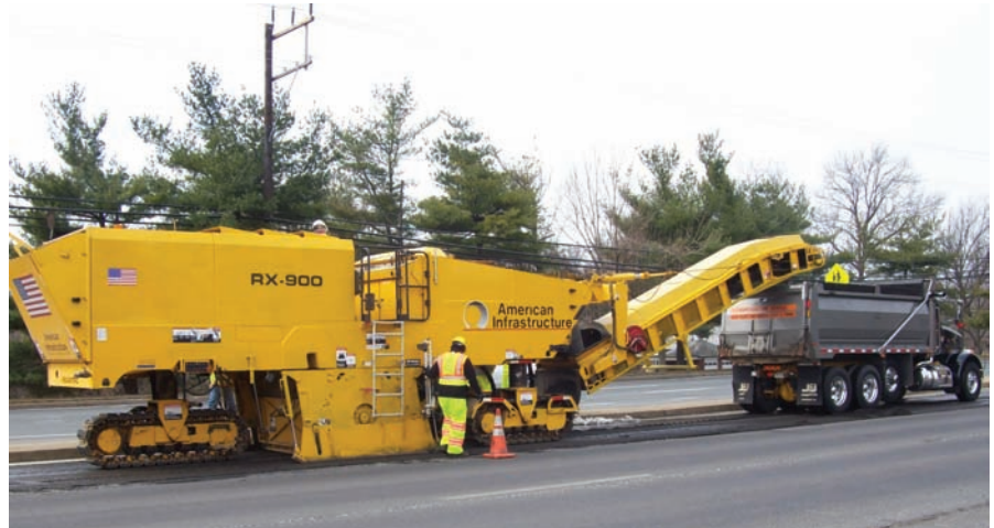
On March 4, Maryland awarded a $2.1-million road resurfacing and improvement project along New Hampshire Avenue in Montgomery County to American Infrastructure. (Photo courtesy American Infrastructure)
